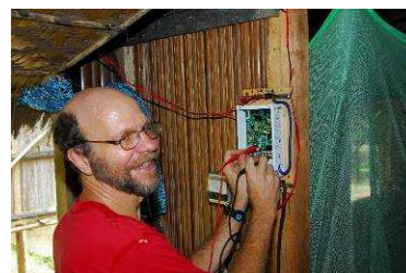
Testing a new installation of a Xantrex C-35 solar controller and two ancient Siemens 55 watt polycrystalline solar panels. A major discovery was the improper gauge wire used to deliver power from the roof that greatly reduced power transfer. West Aitape Multi-Language Project. SIL consultant Beth Fuller's house, North Coast, PNG.
