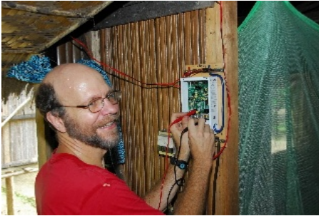
Installing a new Xantrex C-12 Solar Controller in translation consultant Beth Fuller's village house
